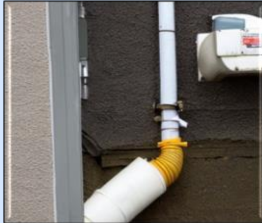
Behind-the-Meter Gas Leaks
