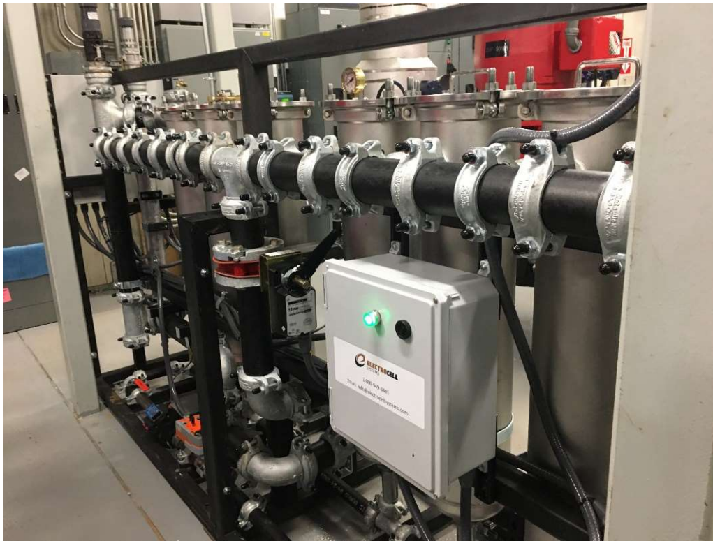
EC-6000 as installed in the 70 NYA chiller plant in Framingham Massachusetts
